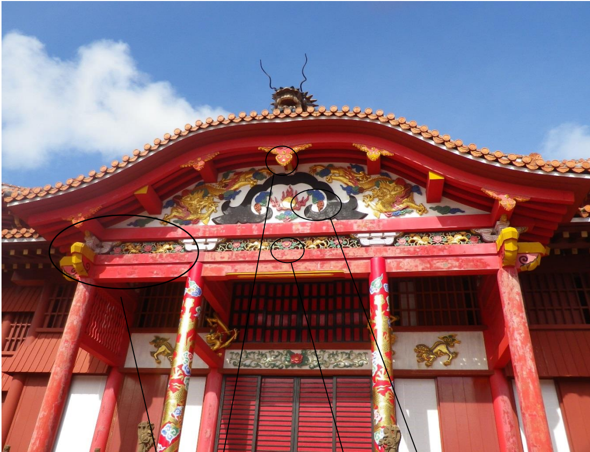
[Condition of deterioration of lacquer coating and vermilion color of the Shuri Castle Seiden and peeling off of gold leaves from the Seiden]
