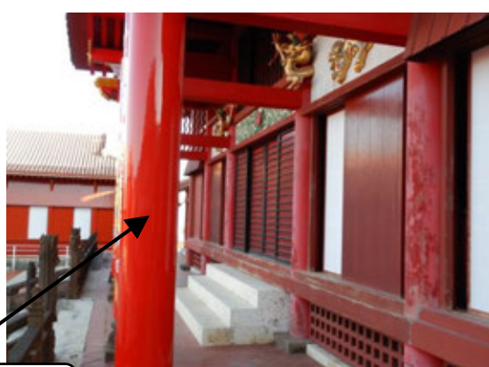
【Kohai inner pillar, doorsill - the lacquer has deteriorated】
